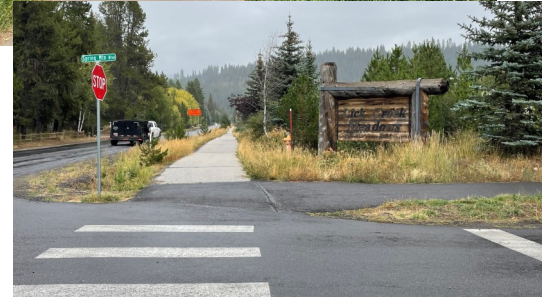
Pathway crossings of streets require detectable warnings and other curb ramps features.
